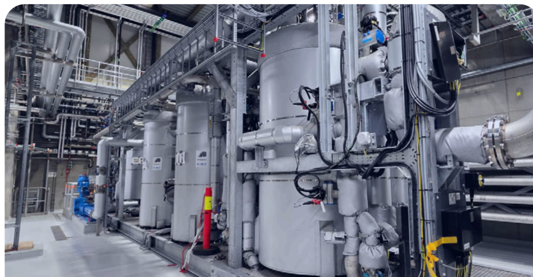
THP system undergoing commissioning in Fredrikstad (Norway)
