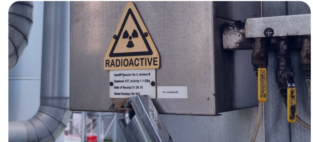
Gamma-source instrumentation is being replaced at older THP sites throughout the UK
